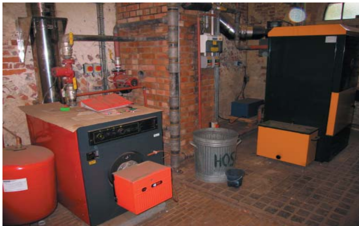
Oil backup boiler, ashcan and biomass boiler
