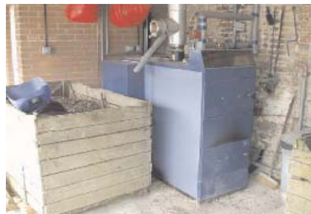
The Baxi Boiler within the woodchip store
