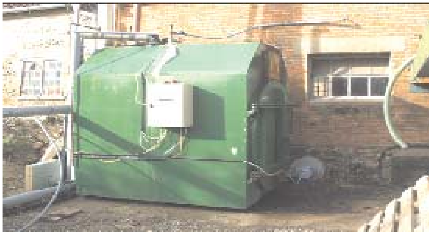
Dragon boiler for grain drying
